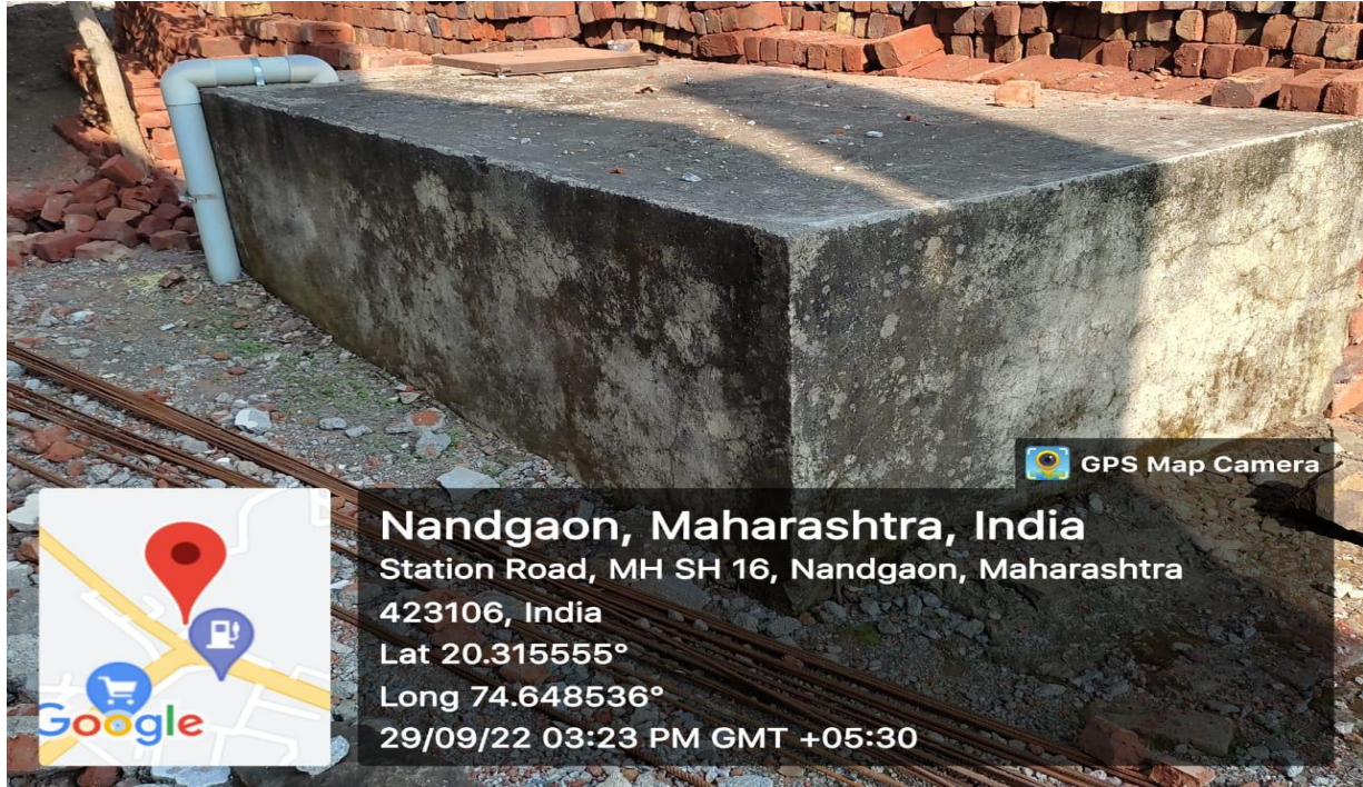
Rain harvesting Tank
