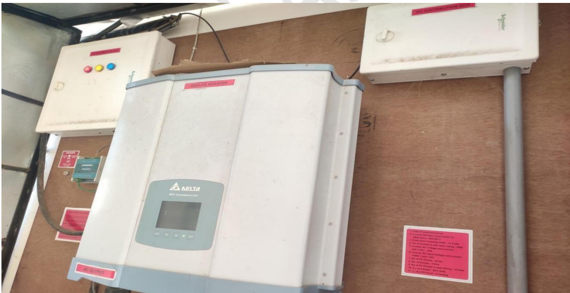
Solar - On Grid Inverter System (15.3KW)
