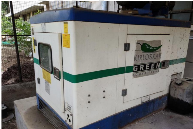
Kirloskar Diesel Generator (15KVA)
