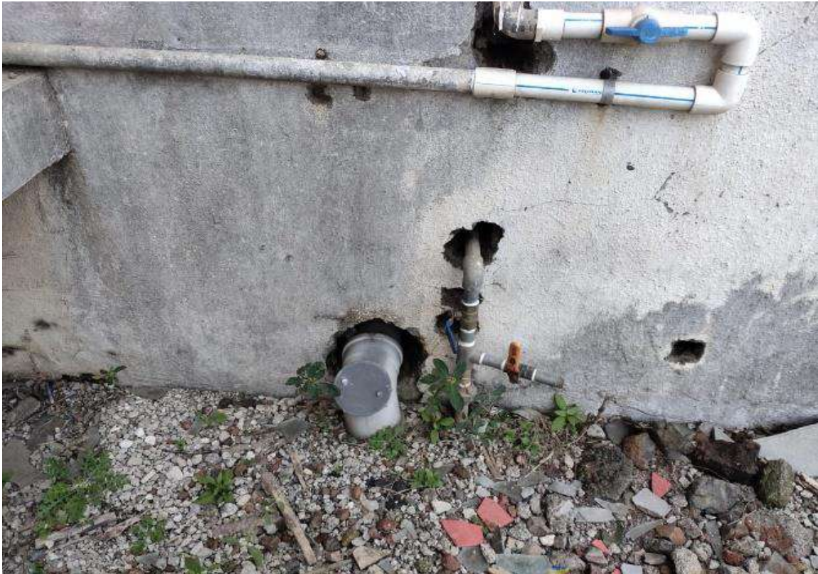
2. Outlet of used chemicals
